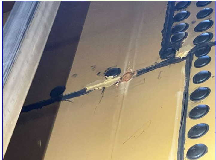
Photo 26 – Interior (June 2022) – View of a caulked plate seam where rust has formed.
