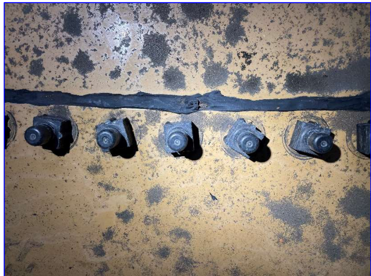
Photo 41 – Interior (June 2022) – View of the sealant used at the tank bottom plate laps.
