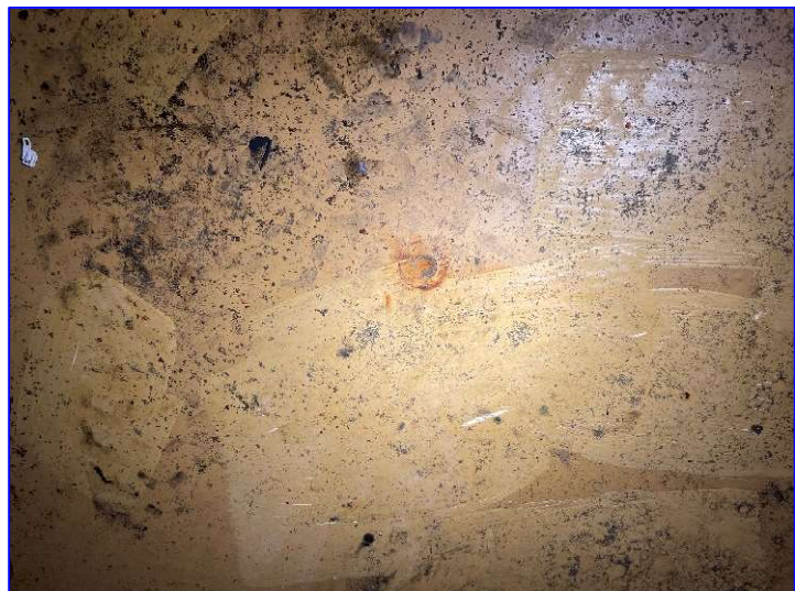
Photo 39 – Interior (June 2022) – View of a site at the tank bottom where a rust nodule has been removed leaving behind deep pitting in the carbon steel.
