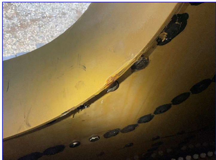
Photo 45 – Interior (June 2022) – View of rust forming at sharp edges of the manway.
