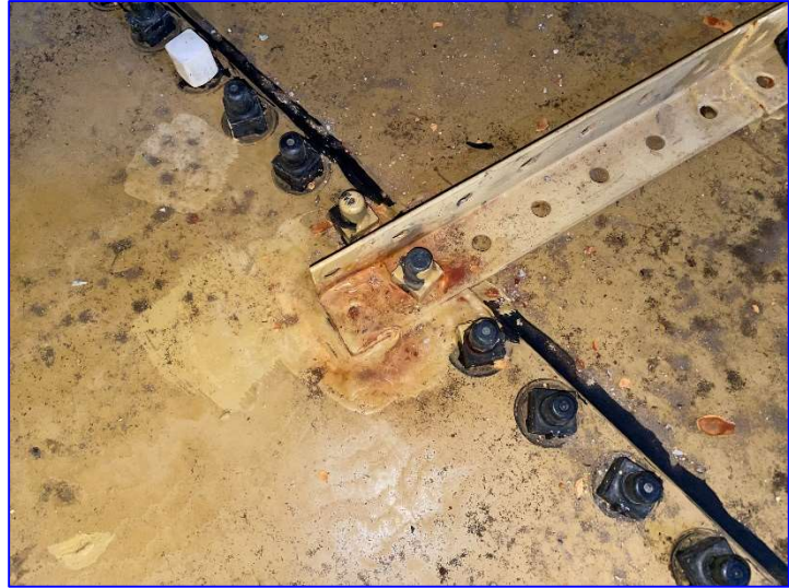
Photo 43 – Interior (June 2022) – View of rust forming at bolt holes of a tank accessory.
