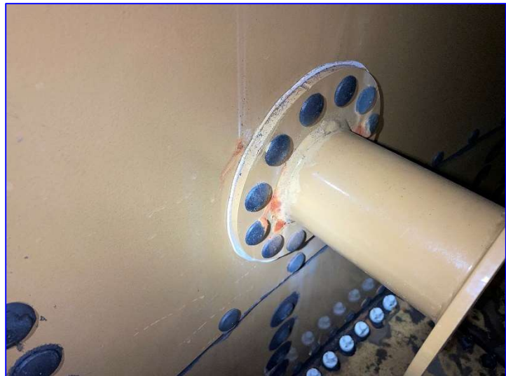
Photo 47 – Interior (June 2022) – View of rust forming at the edges of some capped bolts, accessory flange and piping.
