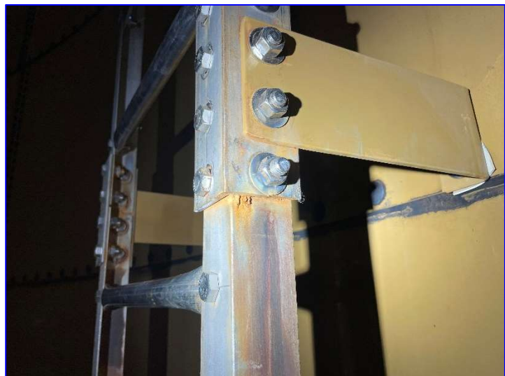
Photo 36 – Interior (June 2022) – View of rust weeping from faying surfaces at the ladder.
