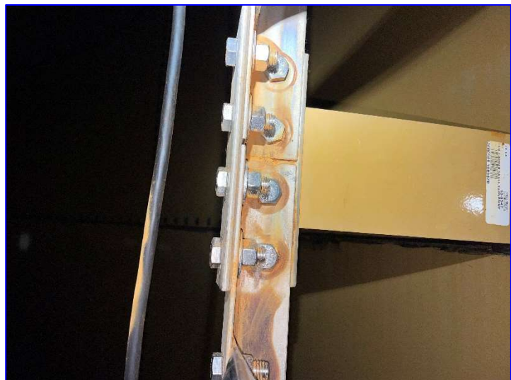
Photo 33– Interior (June 2022) – View of the ladder where stainless steel fasteners mate aluminum to carbon steel and the resulting galvanic corrosion.
