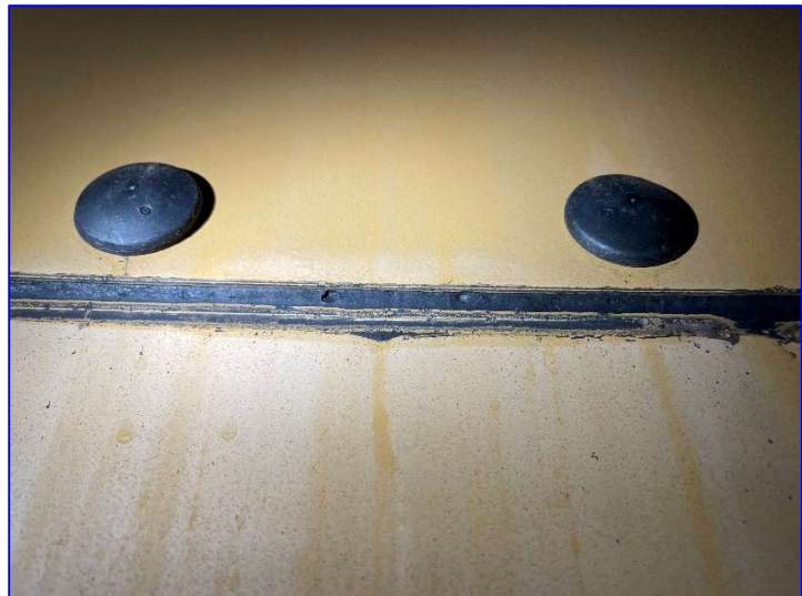
Photo 29 – Interior (June 2022) – View of minor staining at the edge of a shell plate lap.
