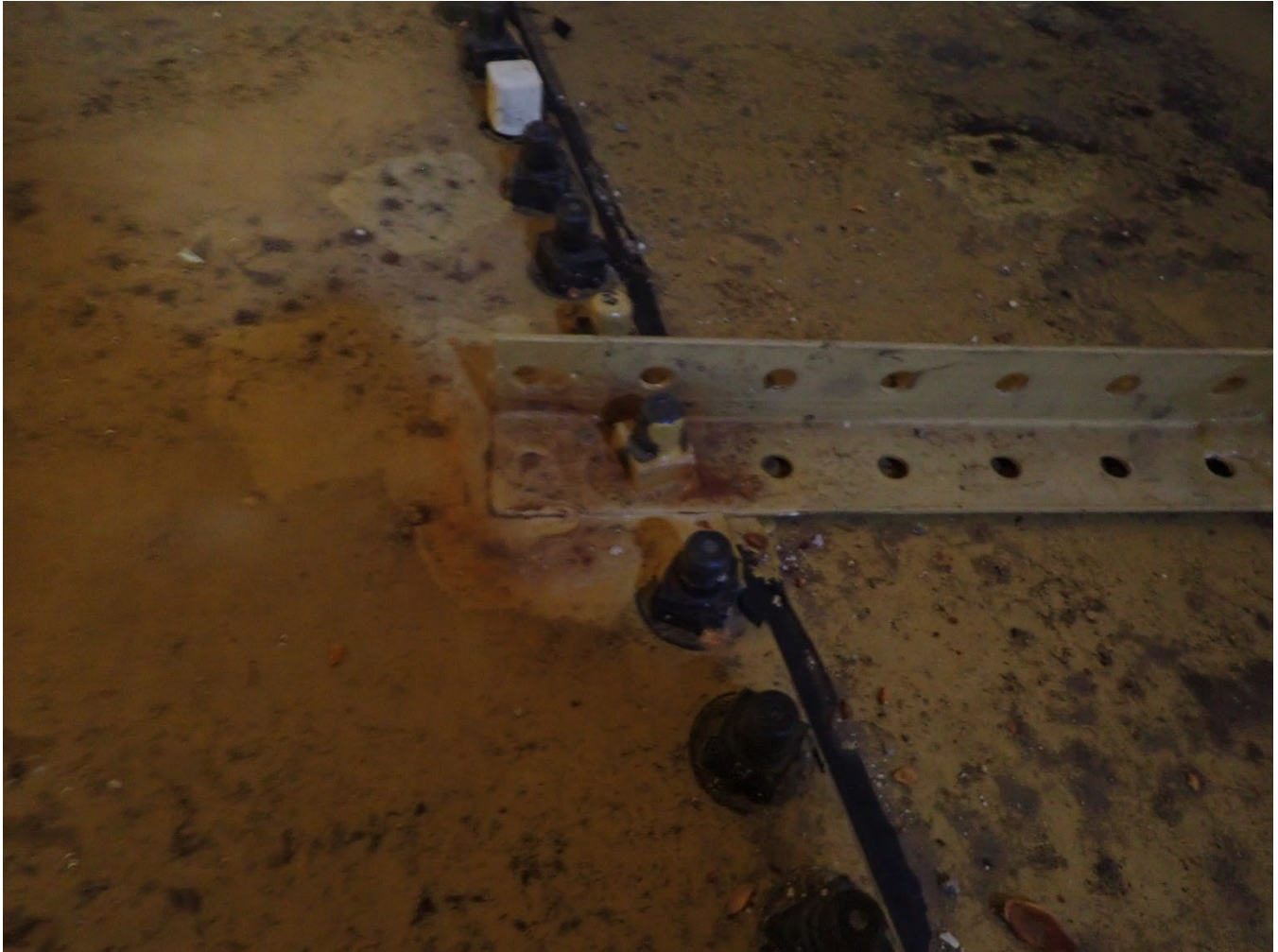
Corrosion at connection of level gauge float support structure
