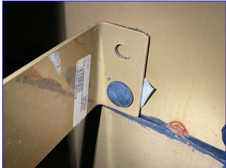
Photo 46 – Interior (June 2022) – View of rust forming at an area of incomplete sealant application
