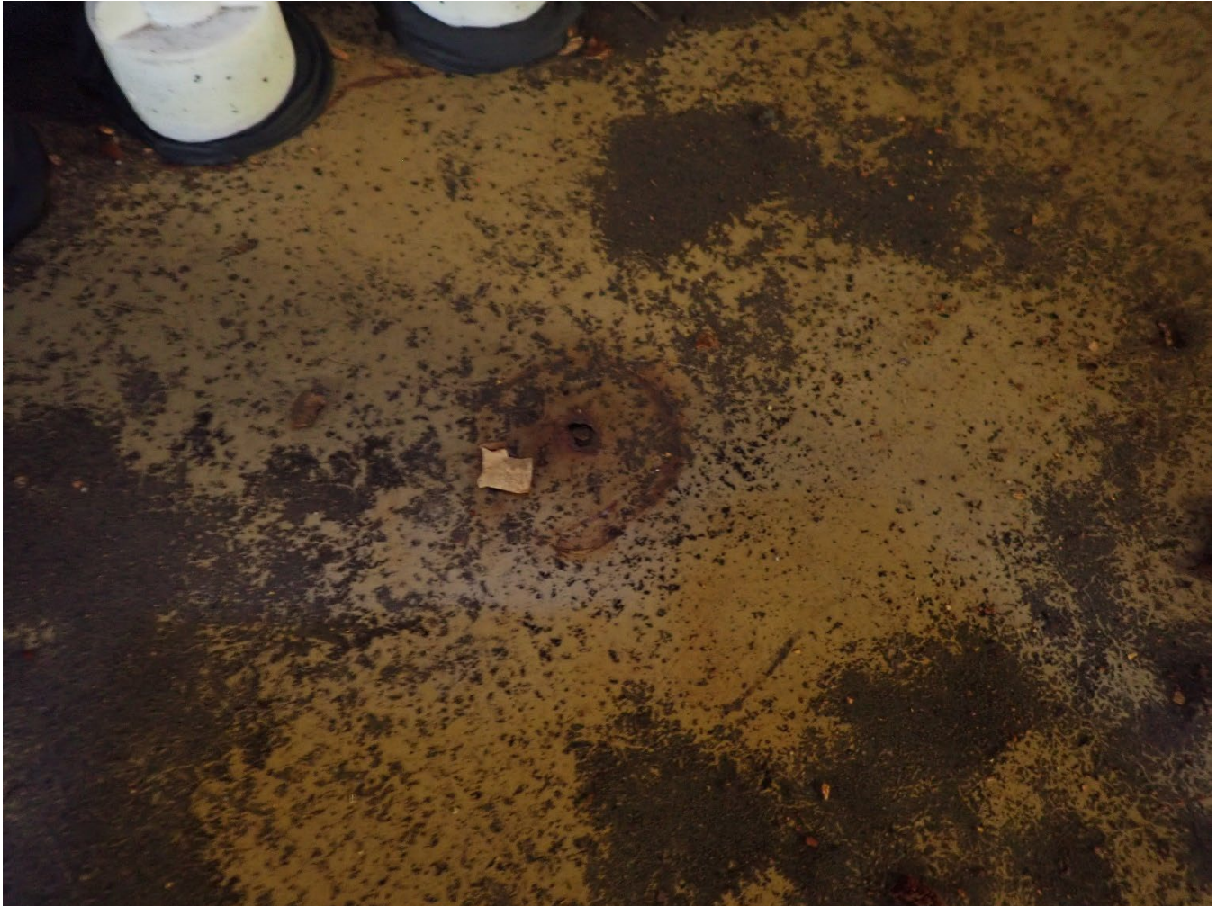
Close up of a rust pit on floor
