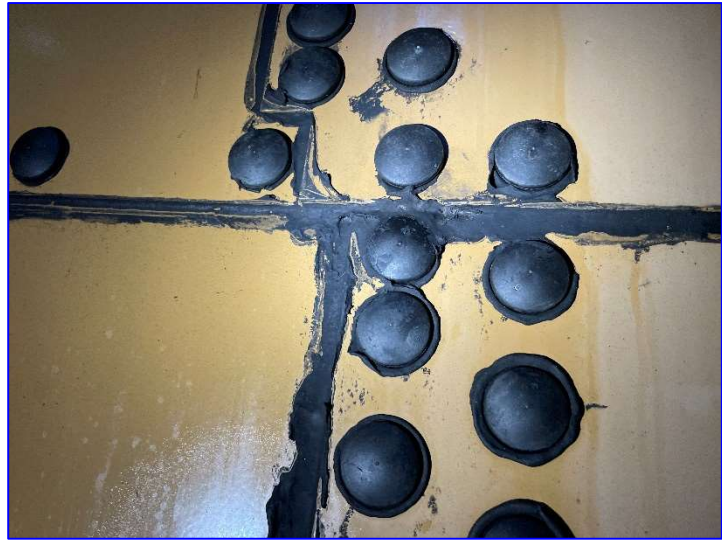
Photo 28 – Interior (June 2022) – View of a plate lap segment of the shell where sealant appears to be performing properly.
