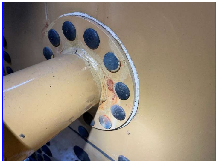
Photo 48 – Interior (June 2022) – View of rust forming at the edges of some capped bolts.
