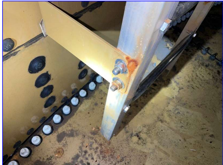
Photo 35 – Interior (June 2022) – View of rust forming at the edges of the ladder stand-offs.
