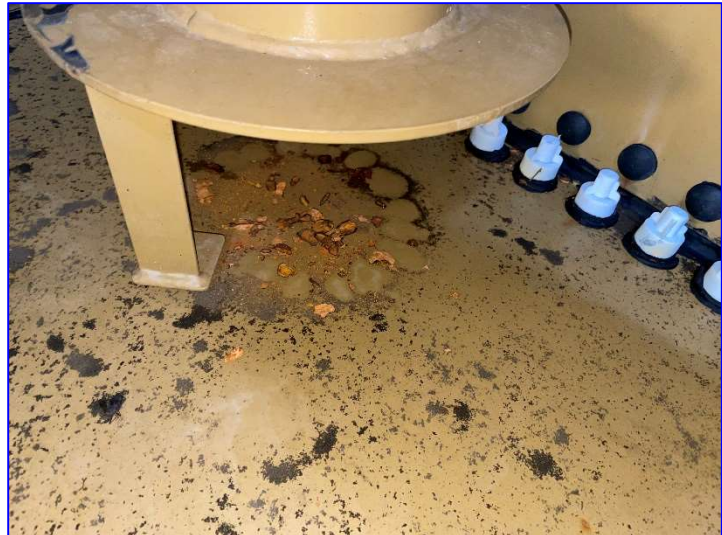
Photo 44 – Interior (June 2022) – View of rust staining from metallic debris.
