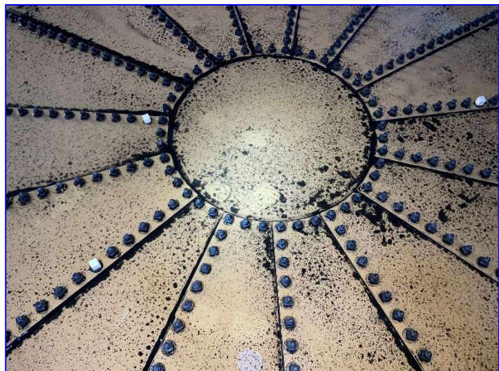
Photo 42– Interior (June 2022) – View of the tank bottom at the center of the tank.
