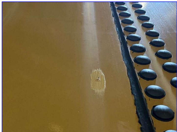
Photo 27 – Interior (June 2022) – View of a lining repair that appears to have failed.
