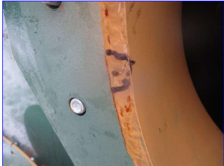
Photo 11 – Interior (Jan 2020) – Shell manway exhibits spot rust at flange mating surfaces.
