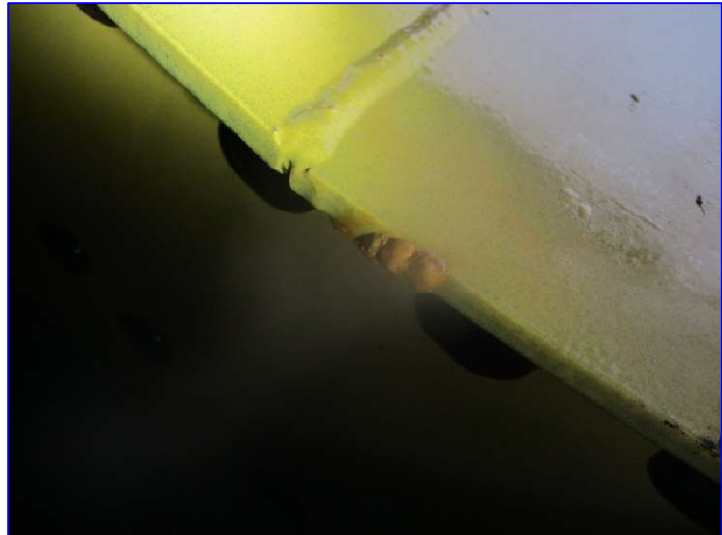
Photo 17 – Interior (Jan 2020) – View of rust nodules at the shell manway.
