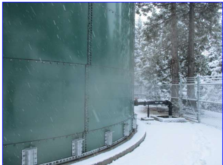
Photo 3 – Exterior (Jan 2020) – View of the lower shell courses and anchorage to the concrete foundation.
