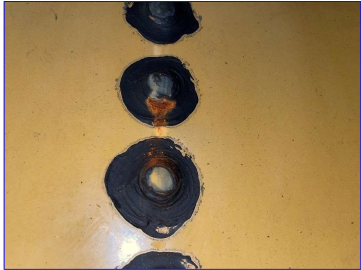
Photo 31 – Interior (June 2022) – View of rust forming at the edges of some capped bolts.
