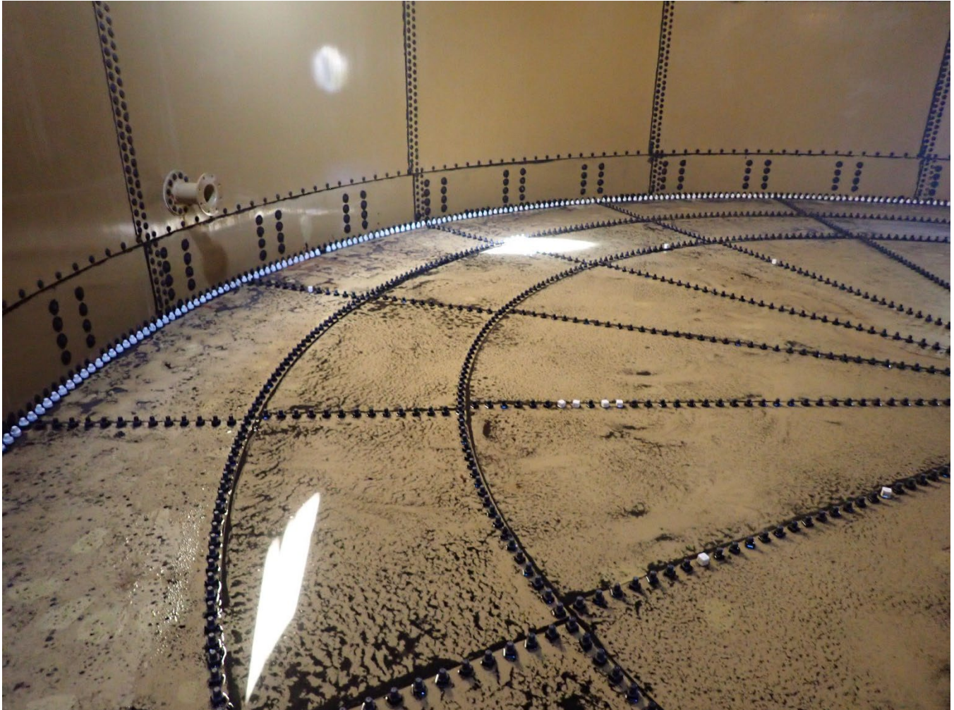
Tank floor with black sediment
