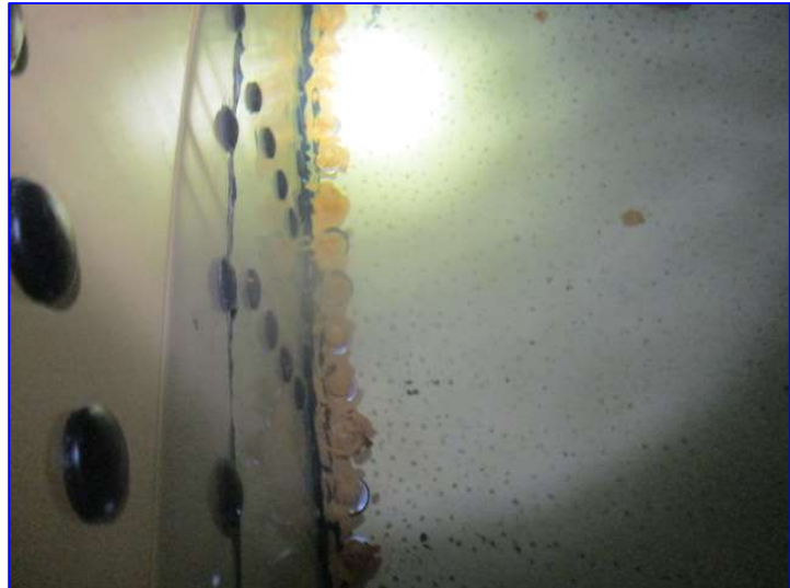
Photo 19 – Interior (Jan 2020) – View of the tank chime where bolts connecting the floor plate to the shell starter ring have developed rust nodules due to the galvanic corrosion between the bolt and the chipped coating at the bolt hole.
