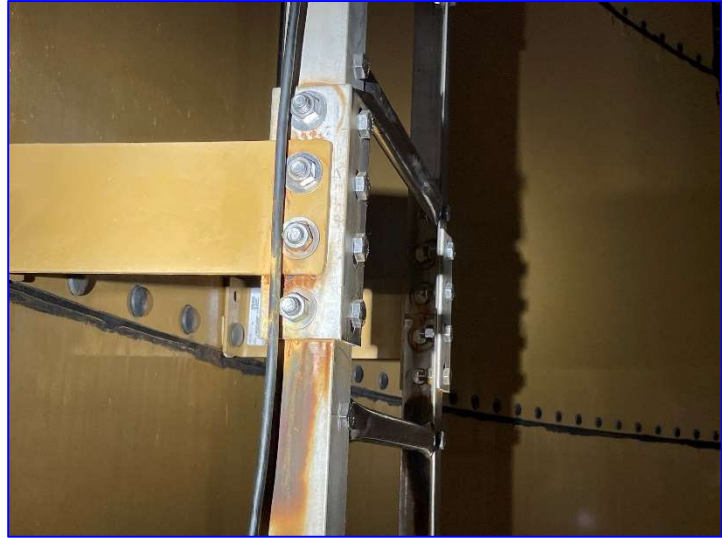
Photo 34 – Interior (June 2022) – View of the ladder where stainless steel fasteners mate aluminum to carbon steel and the resulting galvanic corrosion.
