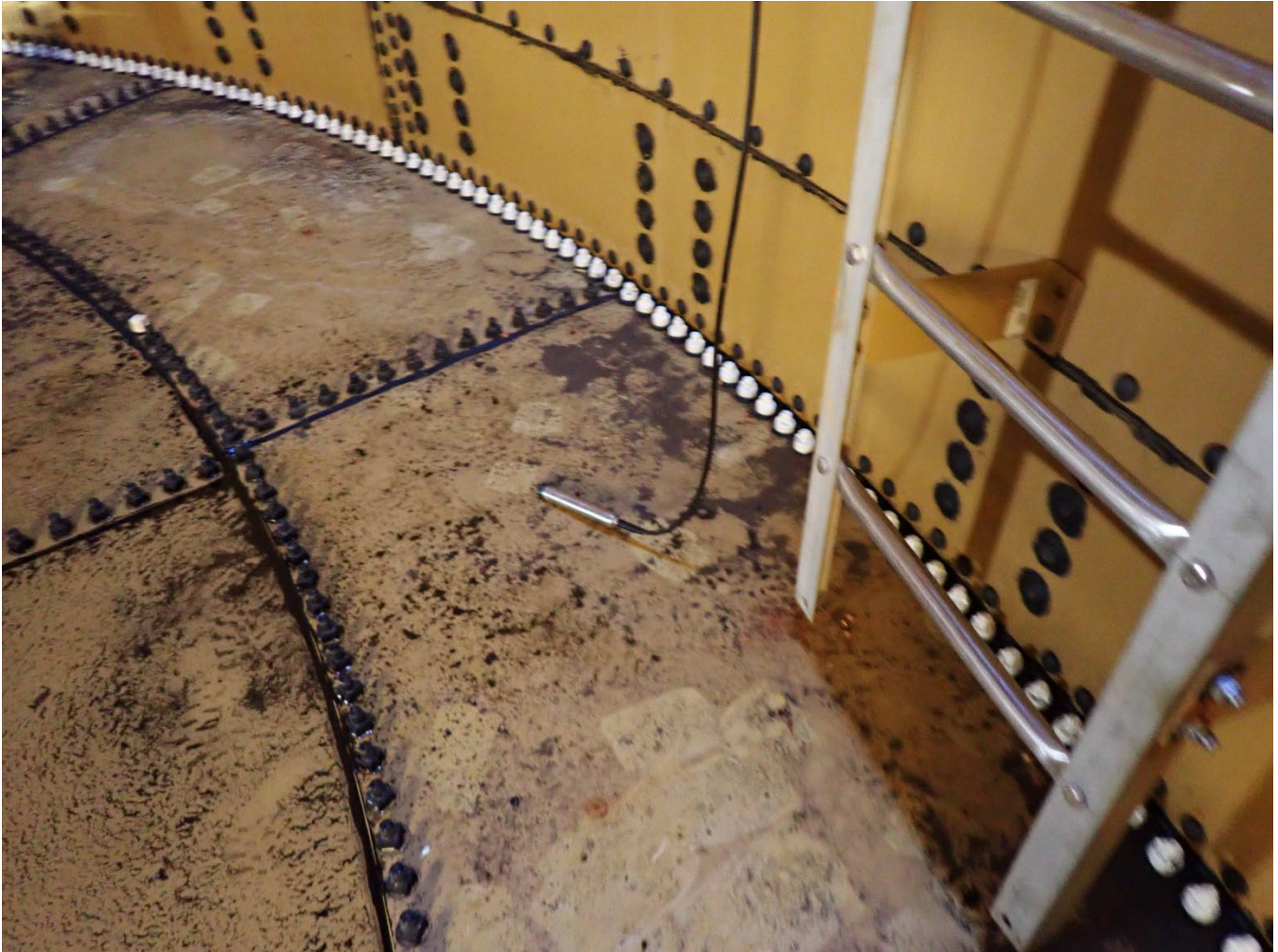
Transducer on floor, rust pits dispersed around and at foot of the ladder
