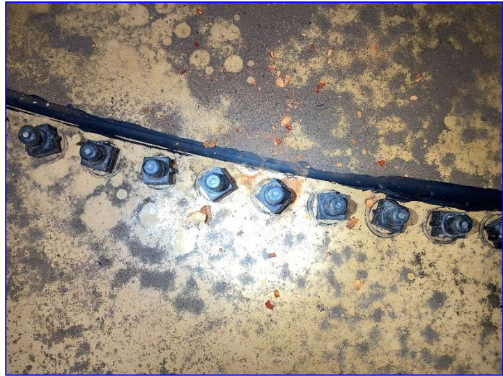
Photo 40– Interior (June 2022) – View of areas of spot rust at the tank bottom, likely caused by mechanical damage.
