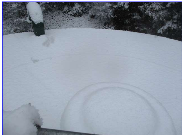
Photo 6 – Exterior (Jan 2020) – Roof surfaces were covered with snow at the time of the inspection.
