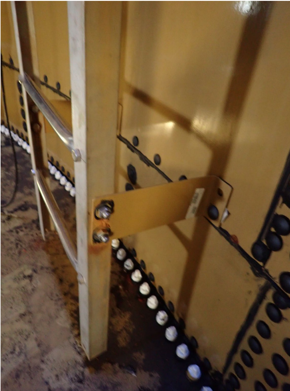
Aluminum ladder with rust at connections and at seam on wall
