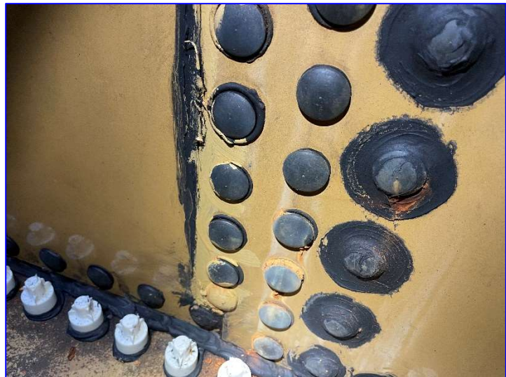
Photo 32 – Interior (June 2022) – View of rust forming at the edges of some capped bolts.
