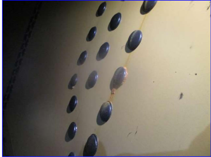
Photo 16 – Interior (Jan 2020) – View of isolated shell bolts where rust has developed.
