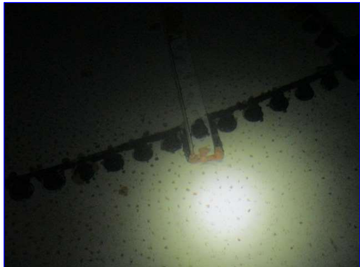
Photo 20 – Interior (Jan 2020) – View of rust forming at the edge of the bolt channel.
